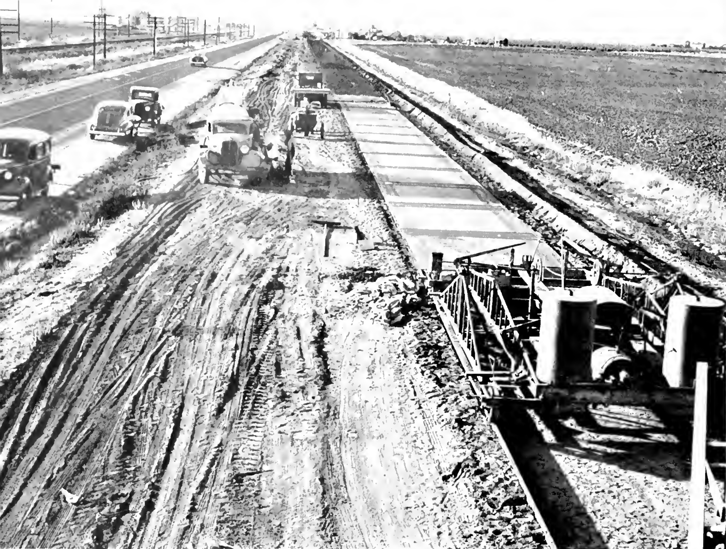
Divided highway under construction between Merced and Chowchilla on U. S. 99. The contract included construction of a bridge over Chowchilla River
